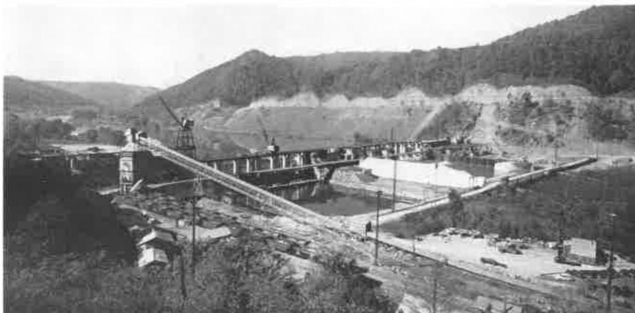
Six sizes of AGGREGATES are delivered from storage bins by a 700-foot conveyor to the CONCRETING PLANT at left above.
